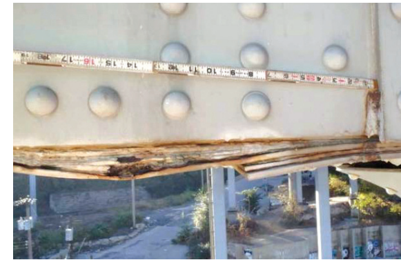
Extensive corrosion at the approach piers
