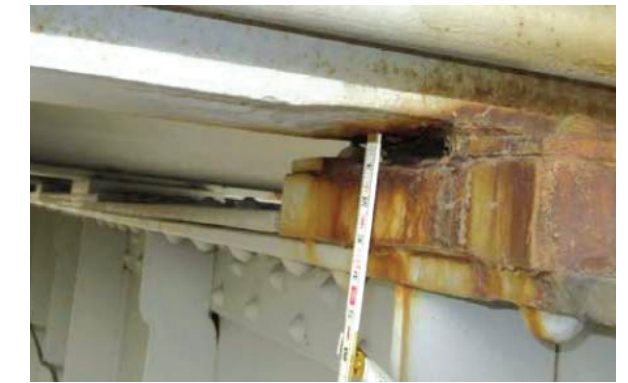
Typical deterioration at steel elements
