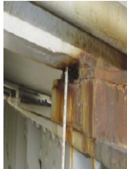
Pack rust at stringer bearing plates
