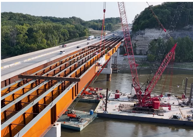
The final girder of the new eastbound bridge is set into place in September.
